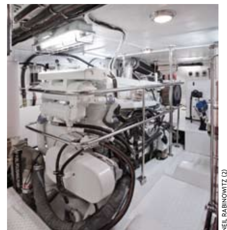
Stainless-steel rails surround the Lugger main engine, which is positioned for 360-degree access.
